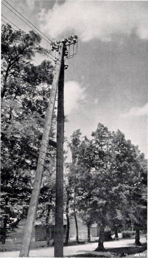
Fig. 3. Method of mounting horn arresters; these are always fixed above the pole to allow the arc to travel upwards out of the horns.
